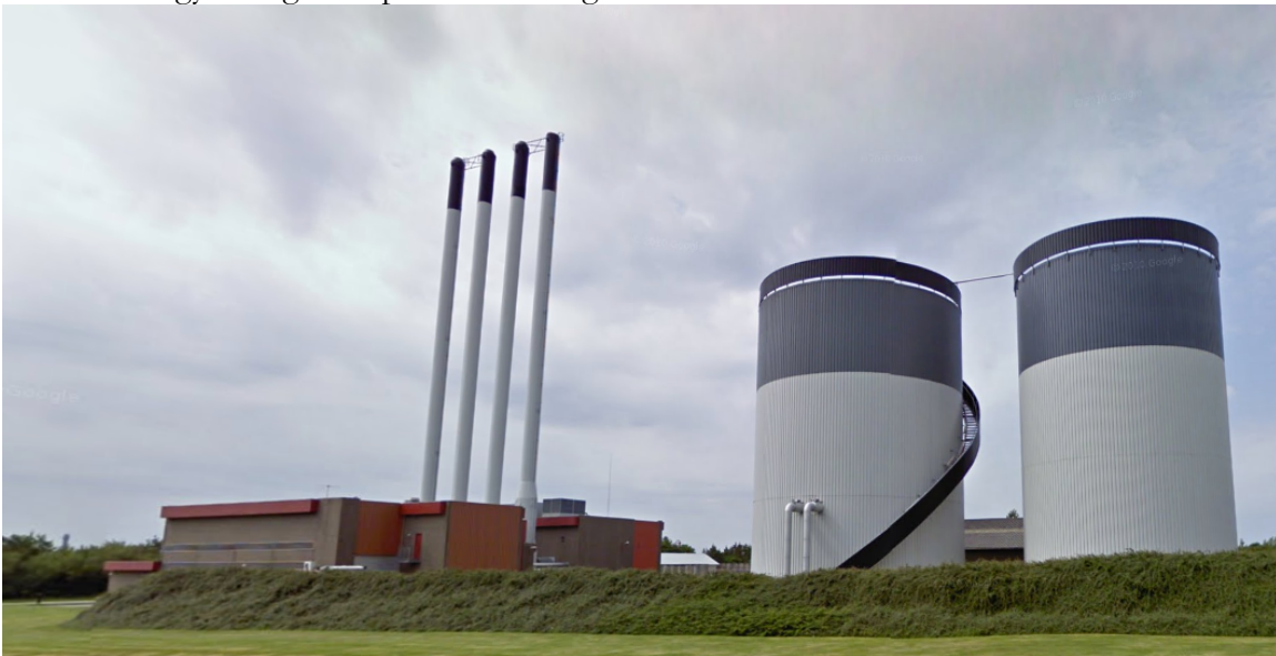
Figure 4 Ringkøbing district heating system hot water storage tanks (at right). The 400 MWh storage capacity system consists of a solar thermal collector system gas boilers, electric boilers, a gas turbine and an internal combustion engine. Waste heat from the turbine and engine contribute to meeting heat demand. The facility can either absorb or generate electric power and stores more than 30 hours of average heat use, or about 20 hours of peak day usage. Source: Google Maps.
